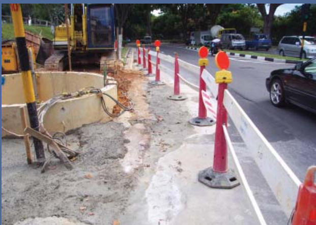
A tell-tale sign of excessive settlement around shafts can be 'making up' the ground as can be seen here with the fresh concrete screed adjacent to a shaft in Singapore.
