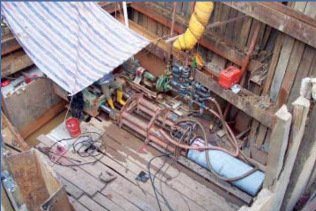
A 300mm ID jacked concrete coated ductile iron water pipe being launched in Singapore.
