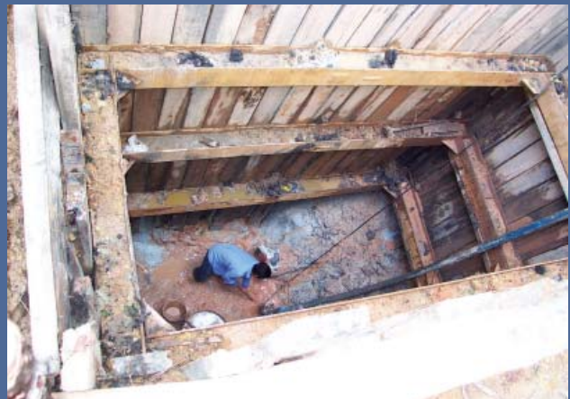
This pipejacking machine in Singapore hit a boulder and because it had no cutting discs a rescue shaft needed to be excavated in order to then relaunch the machine.
