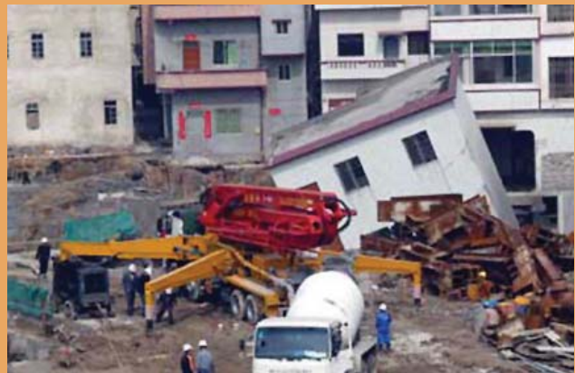
1 April 2004 – Collapse of building caused by construction of Shanghai Metro.
