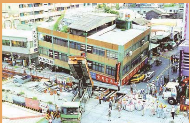
9 August 2004 – Underground construction of Kaohsiung MRT in Taiwan caused sinking buildings.
