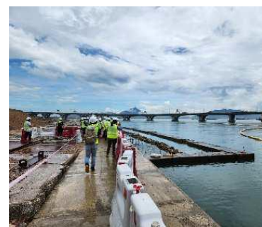
Viewing of the eco-shoreline with mudflat, mangrove, and oyster baskets. Silt curtain was also observed surrounding the site as an environmental protection measure.
