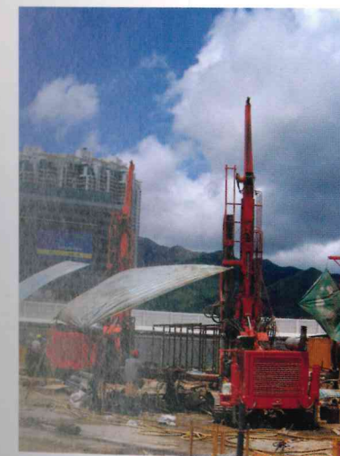
Plate 1.2. Drilling rigs at a development site on a reclamation close to the new international airport, Lantau Island
