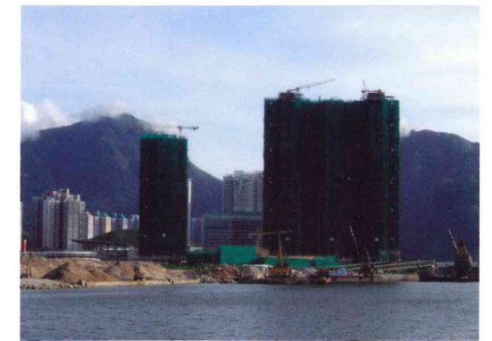
Plate 2.1 Apartment blocks on a reclamation site at Tung Chung, Lantau Island. The mountains in the background are composed of volcanic rocks. These are faulted against metasedimentary rocks and granite, which underlie the reclamation and offshore areas. Alluvium and marine deposits blanket the seafloor.
