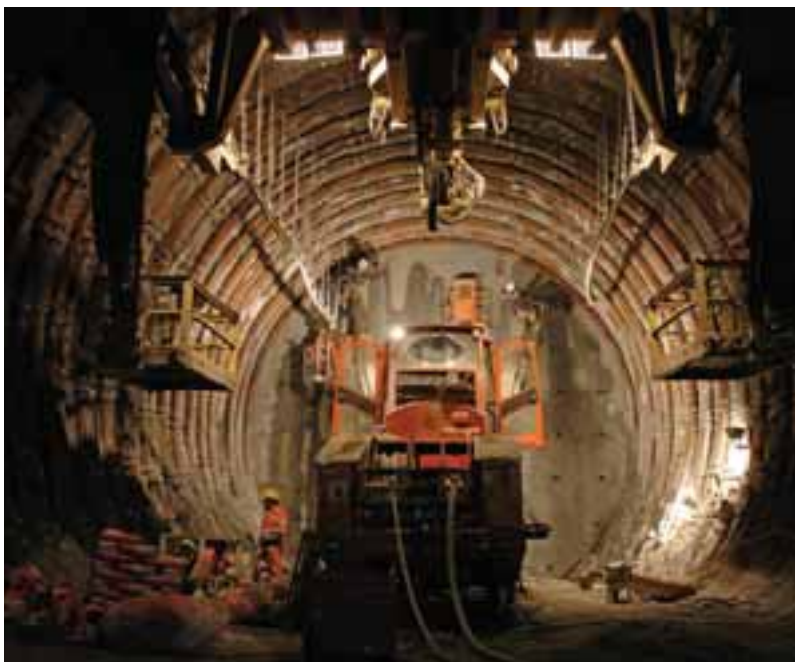
Excavation work with conventional tunnelling in squeezing rock conditions, Sedrun northern drive.
