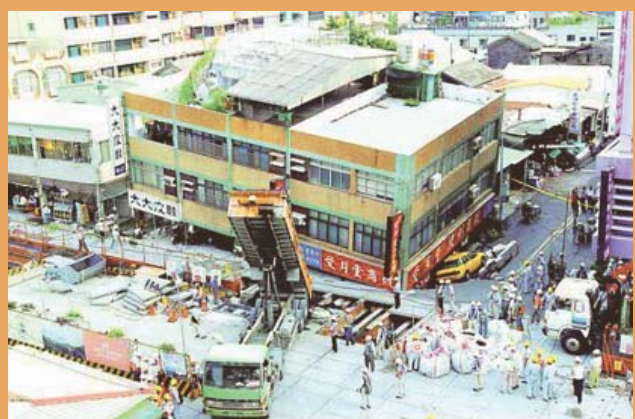
9 August 2004 – Underground construction of Kaohsiung MRT in Taiwan caused sinking buildings.
