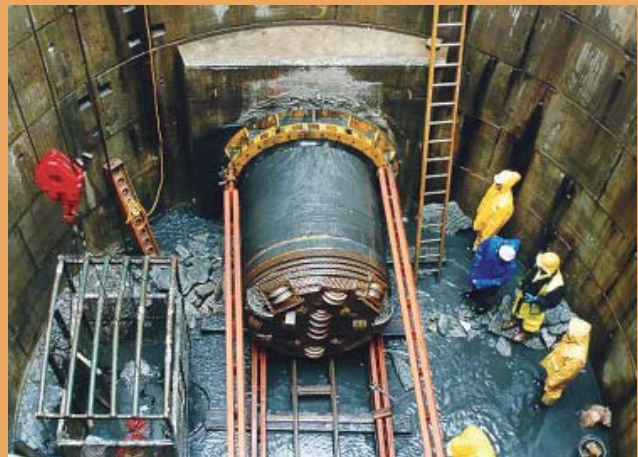
A pipejacking machine suitable for rock excavation is entering a reception shaft through a watertight collar in the UK.
