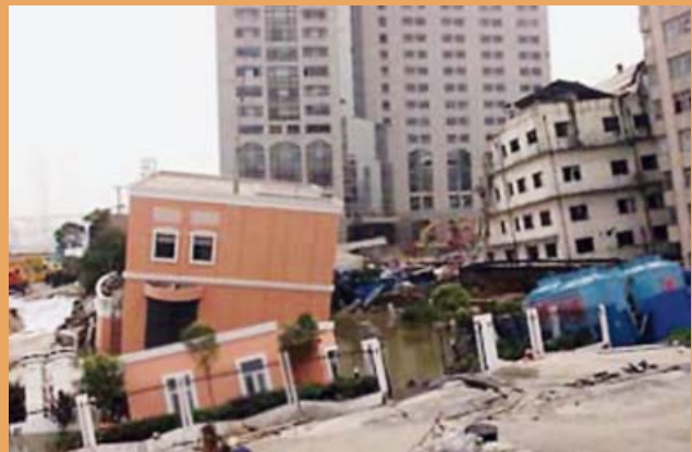
1 July 2003 – Tunnelling Works for Shanghai Metro caused massive subsidence and structures requiring demolition.
