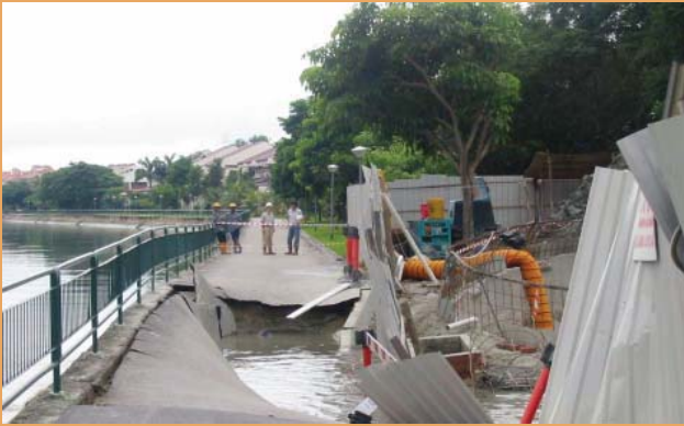
In Singapore a shaft collapse can be seen adjacent to a canal which in turn induced flooding in the shaft.
